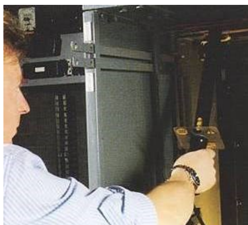
HVI - Switchgear Testing
